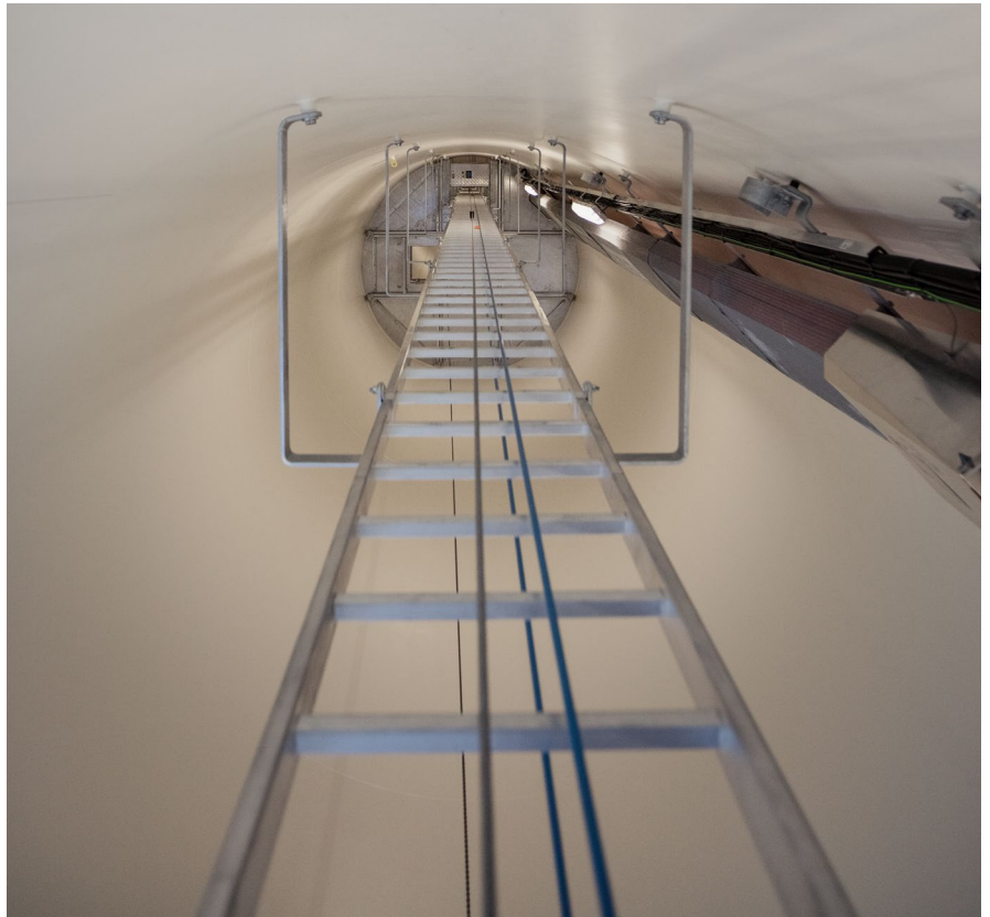
Interior of turbine at Golden Hills wind farm in California (43 MW for Google)
